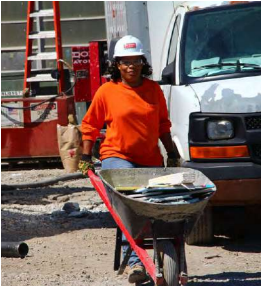
A worker pushes a wheelbarrow at the site of the Dunne Technology Academy modernization project.
