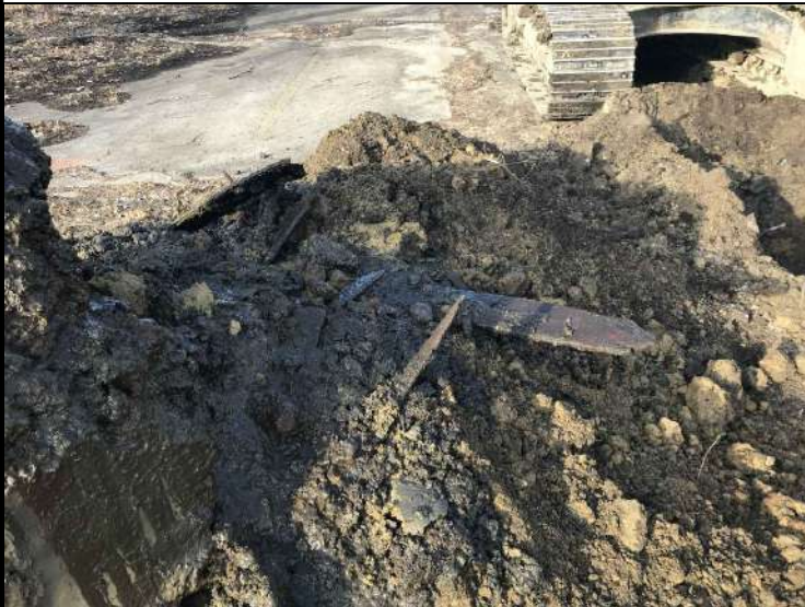
15: TP-13, building debris
