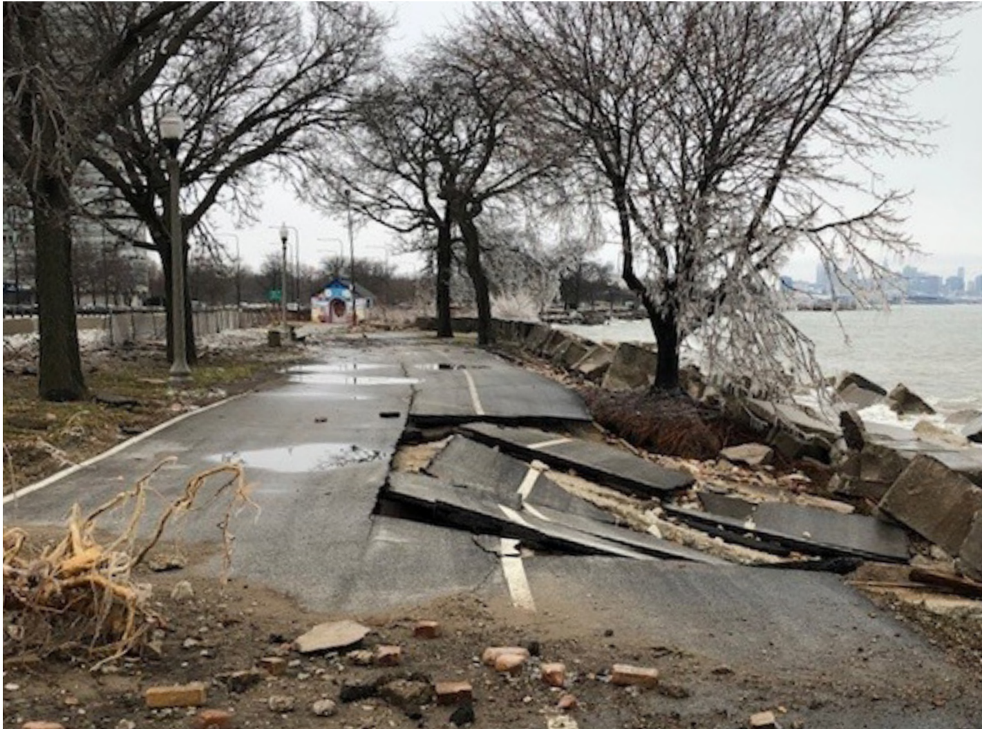
Storm damage resulting from inadequate shoreline protection, January 2020.
