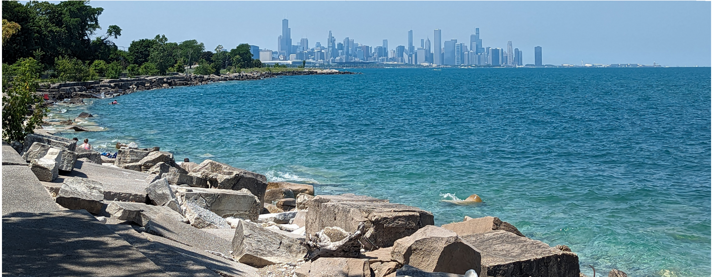
Existing edge of lakefront trail crumbling into the water limits areas where park visitors may safely interact with the lake.
