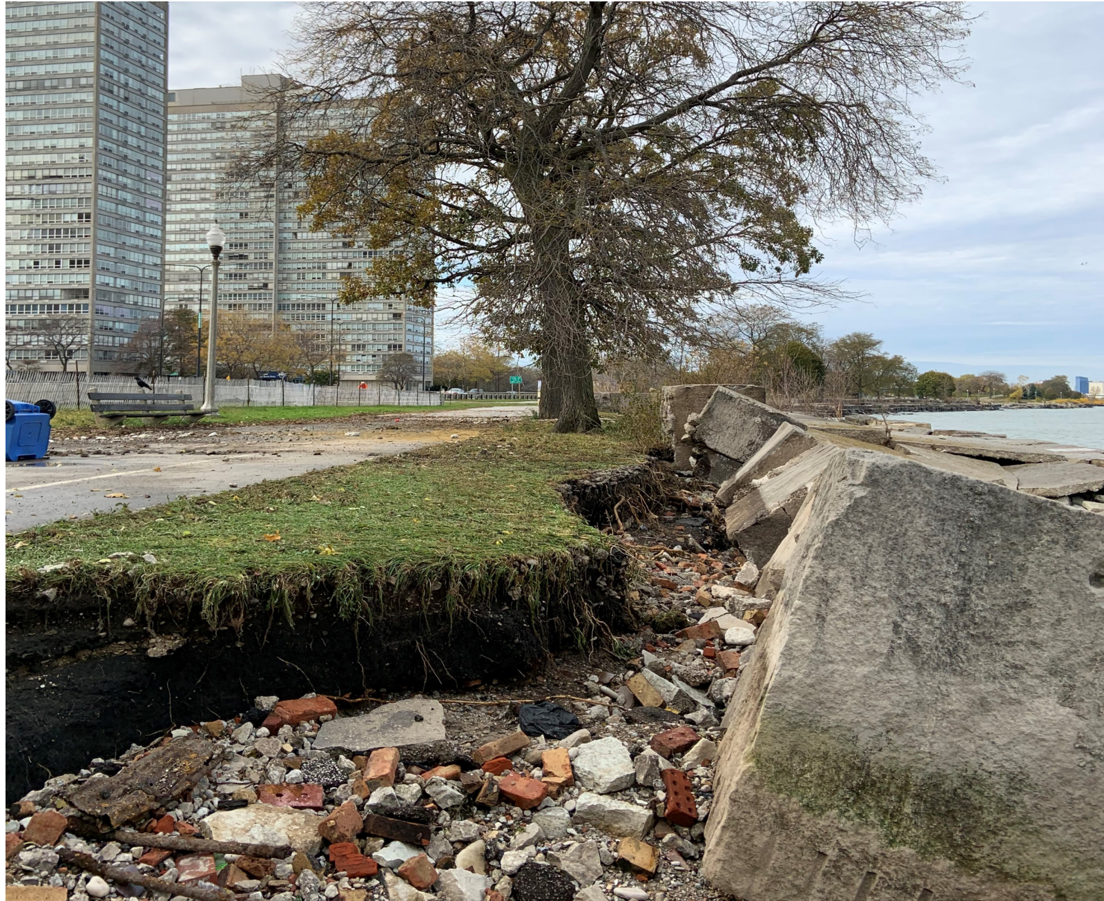
Dislodged revetment stones and parkland erosion due to wave action.
