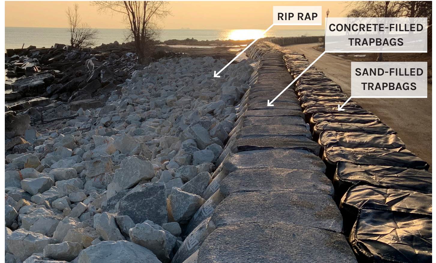
Deteriorating shoreline separated from pedestrian trail with temporary measures of rip rap and TrapBags.
