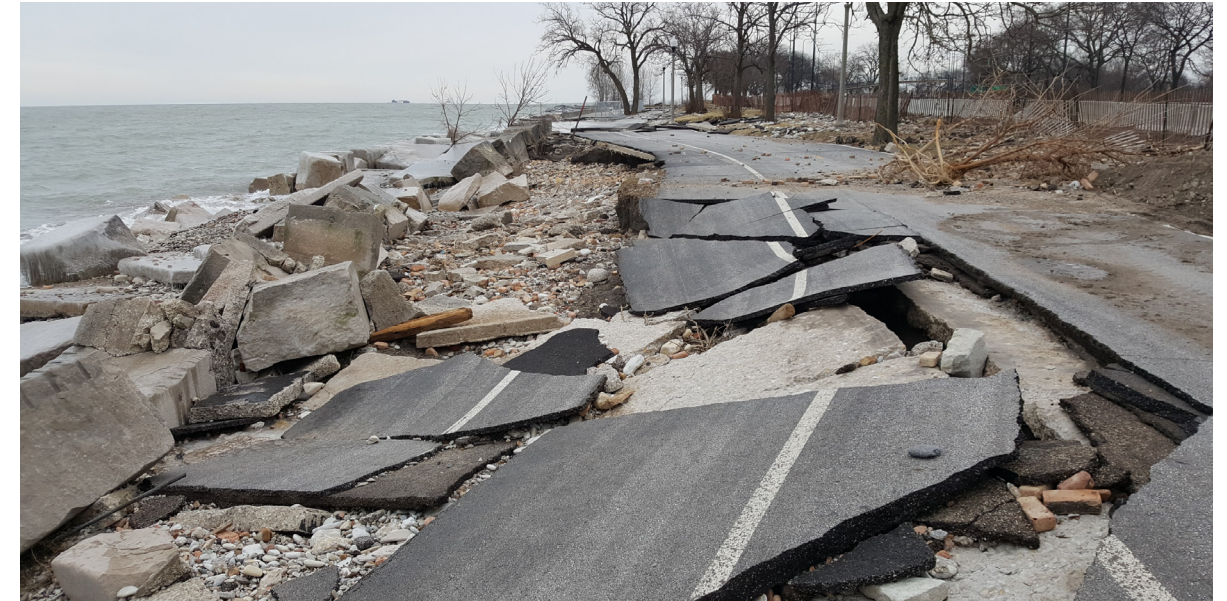
Destroyed lakefront path due to wave action.
