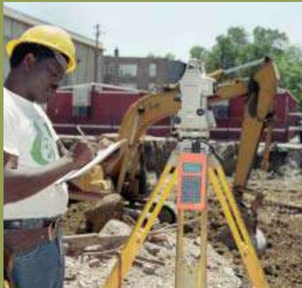
Pre-construction activity at the future site of the Edward "Duke" Ellington School
